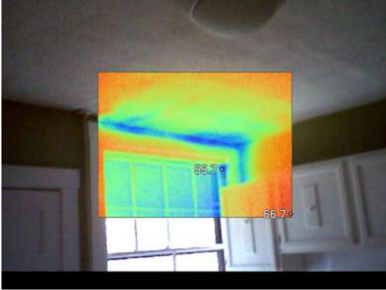
Air Infiltration above kitchen window.
